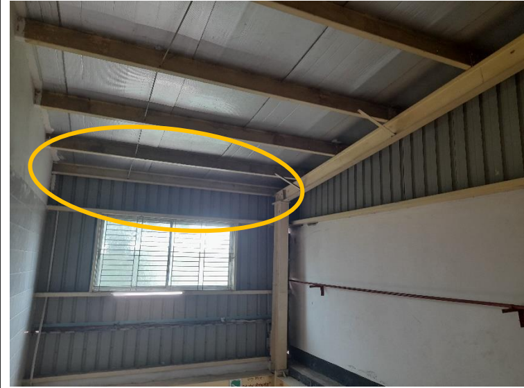
Compression strut missing in gable frame
