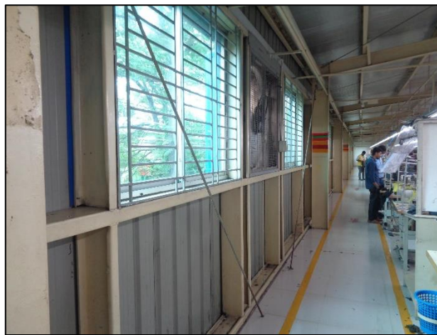
Cable bracing (1st Floor)
